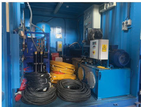
Quincy LP Compressor / HP Compressor / Hydraulic Power Pack 30HP
