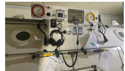
DDC Control Panel
