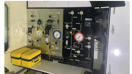
Dive Control Panel
